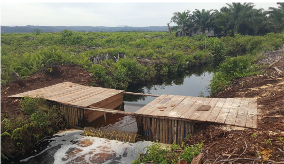
Figure 3-26: Center overflow in timber box block to allow small boat to pass through (Source: Ministry of Environment and Forestry, Indonesia) (Note: Low level of this spillway means the upstream peat is not fully rewetted).
