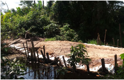
Figure 3-16: An Earth-fill Block made of wood, soil bags and earth fill in a medium-width canal
