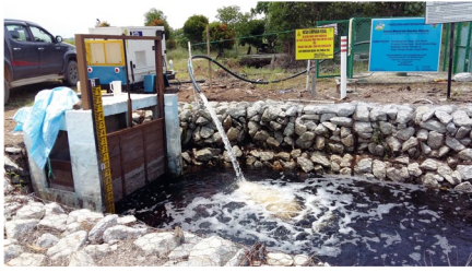
Figure 3-22: Gabion and watergate with water being supplemented by adjacent tube well (Note: Gabion structure, with large rocks, is not appropriate as it lets water pass through the rocks and bypass the gate)
