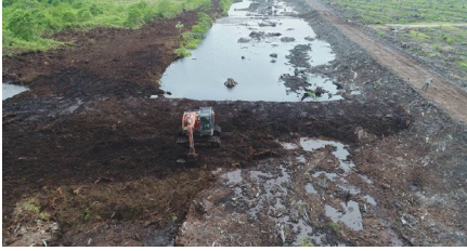
Figure 3-12a (left): Compacted peat dam constructed in series of 5 along the 20+ metre-wide canal along the western side of the Tahura OKI (buffer zone of Berbak NP); these were constructed in the wet season Jan-Feb 2018 and were functioning well after 1 year (Photo courtesy of Mott MacDonald).
