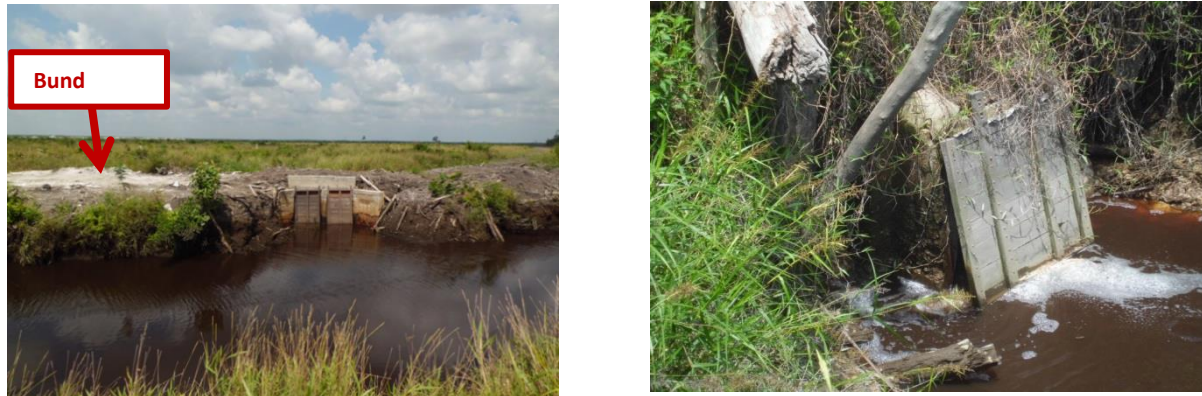
Figure AP3-2. System with Bund and Flap Gates. The Flap Gates closes automatically during high tide, preventing influx of tidal water (Left). The Flap Gates open automatically during low tide, allowing drainage (Right).
